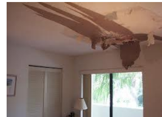
Ceiling Leak Damage
