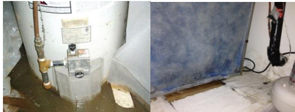
Water Heater & Air Handler Leaks
