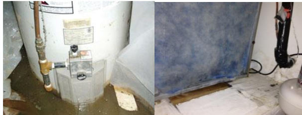
Water Heater & Air Handler Leaks
