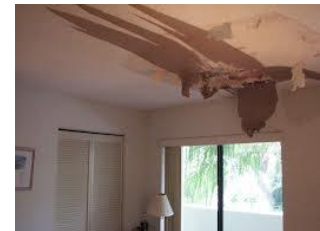
Ceiling Leak Damage
