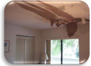
Ceiling Leak Damage
